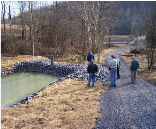
Figure 2. Water gains alkalinity as it flows through a leach bed at Site 3
